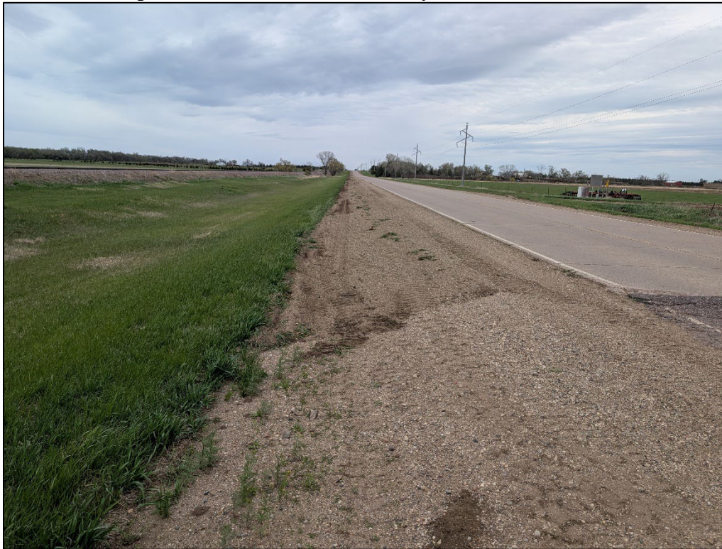
05-04-2026 Impacted Shoulder And Roadway West Of Above Photo
