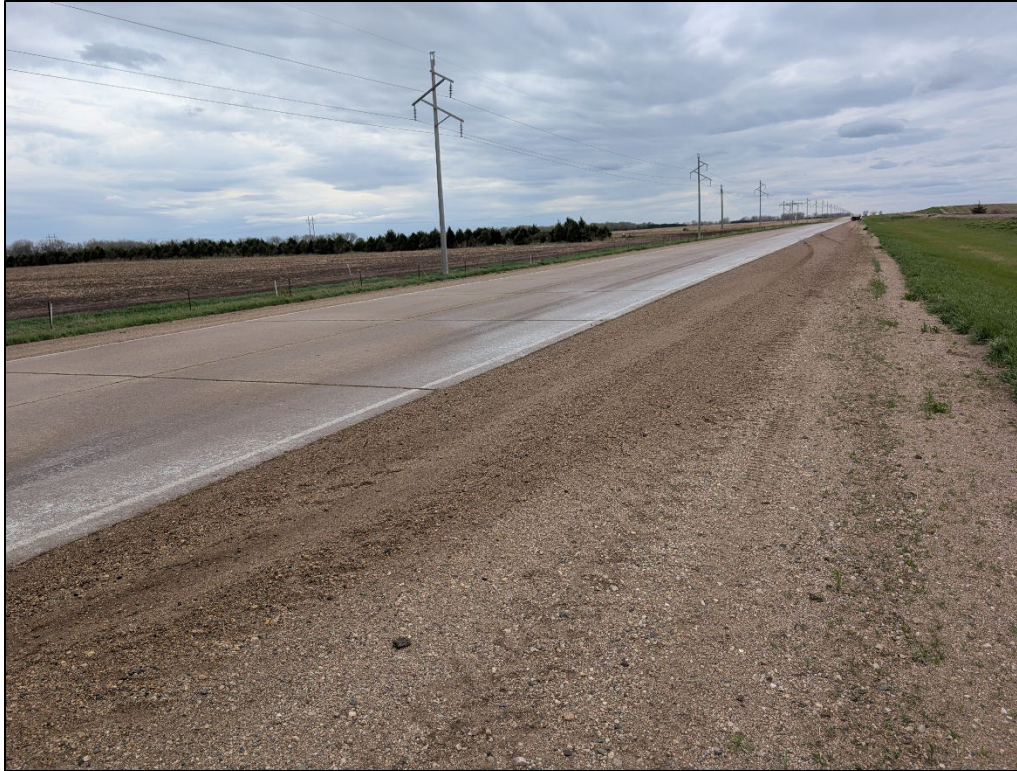
05-04-2026 Impacted Roadway Looking East
